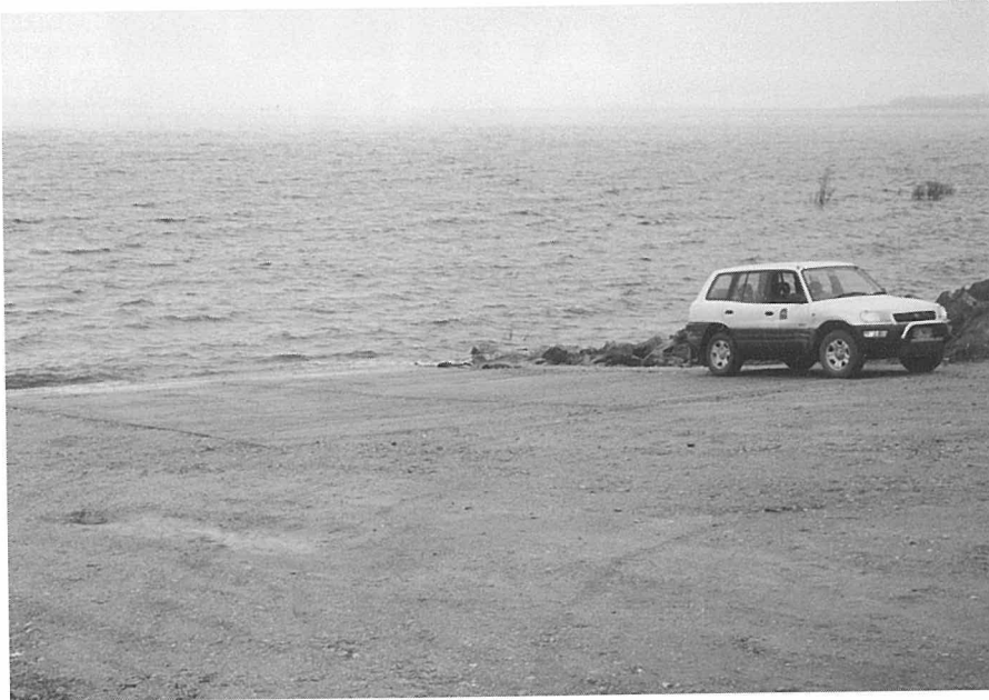
Double width concrete addition to the boat ramp at Brandum Bay, Great Lake
